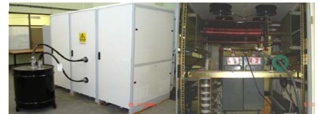
Figure 4 left: resistive load in oil tank (@110kv) connected to modulator; right: bouncer circuit elements pictures at RRCAT
