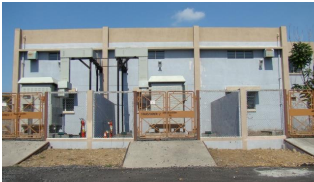
Central Complex Sub-Station
