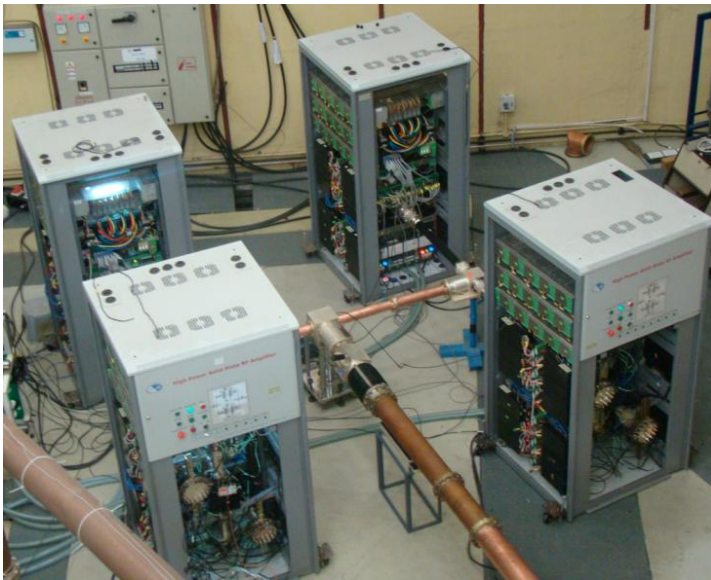
Indus-2 RF station with solid state amplifiers (75 kW)
