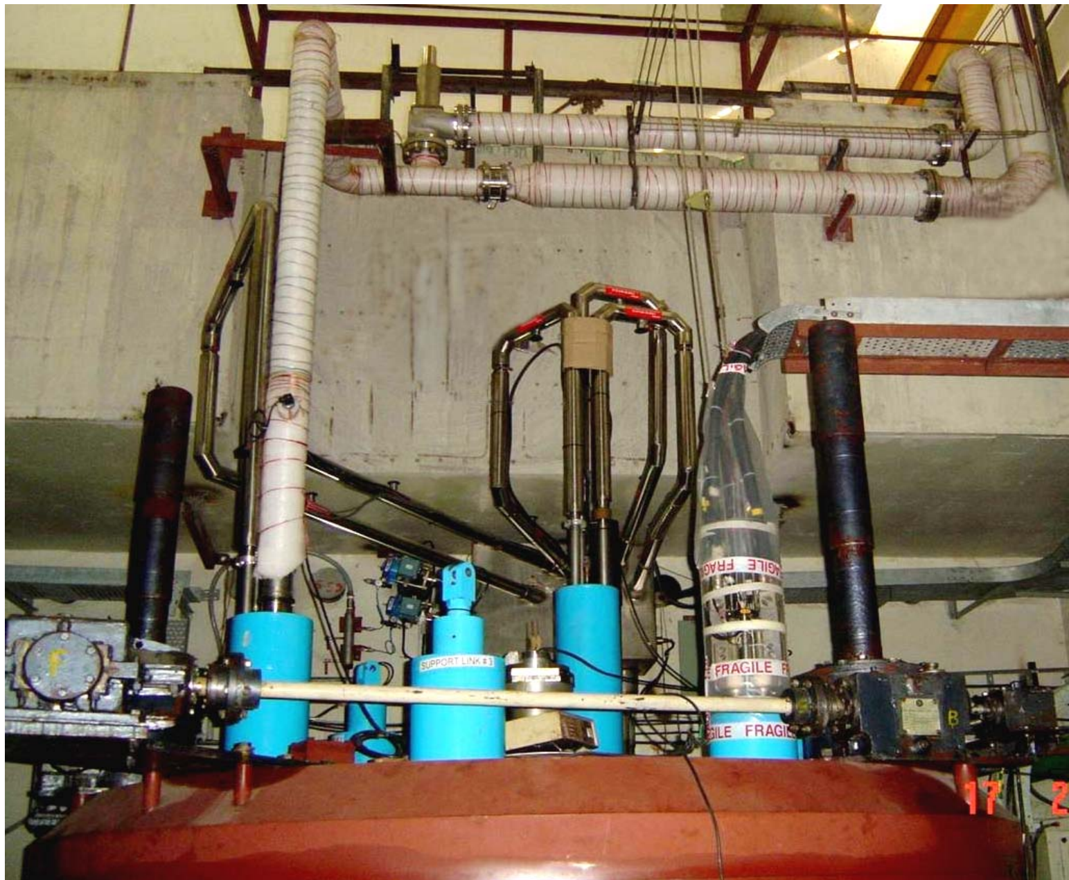
Transfer lines connected to the SC magnet
