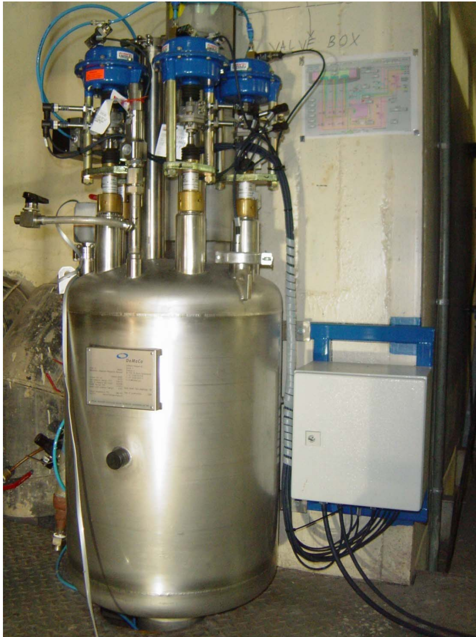
Basement mezzanine manifold for supplying liquid nitrogen to the magnet cryostat
