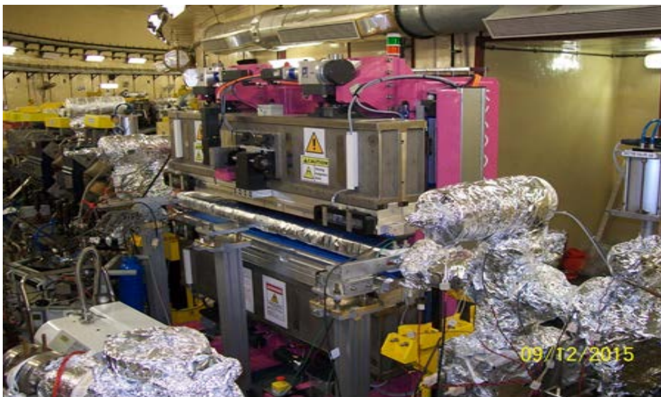
Fig. 2: APPLE-2 undulator installed in LS-5 along with the compatible vacuum chamber and other peripherals.
