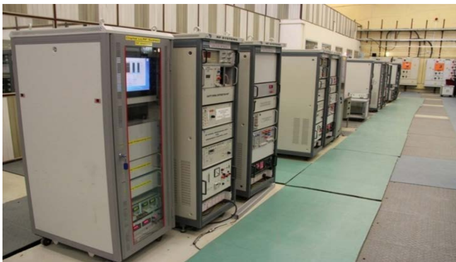
Fig. 21: Digital LLRF systems installed with four RF stations in Indus-2.
