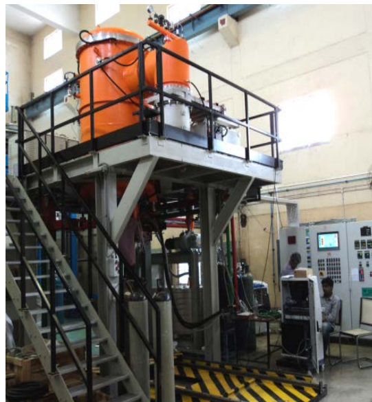
Fig. 27. The controlled atmosphere brazing furnace
