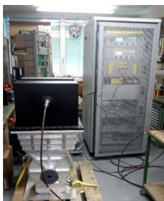
Fig.VI.1.1 : 20 kW Solid state power amplifier.
