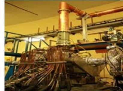
Fig.I.B.2: RF Cavity installed and connected to RF power station through transmission line .
