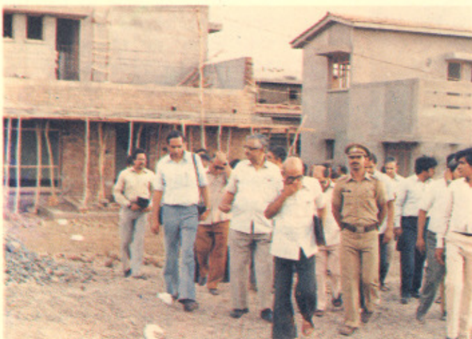
May 1985—Dr. R. Ramanna visiting the construction site of housing complex of CAT. To his right is Dr. D.D. Bhawalkar and to the left Shri C. Ambasankaran.
