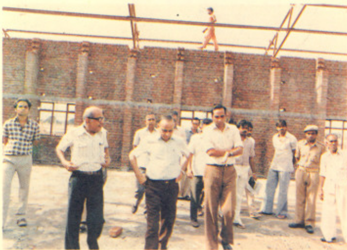
July 1985—Dr. P.K. Iyengar, Director, BARC at the construction site of Multipurpose Shed at CAT. Seen to his left is Dr. D.D. Bhawalkar and to the right Shri C. Ambasankaran.
