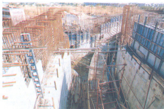
Radiation shielding walls of Indus-2 building. In the center is the magnet foundation, also seen at the middle is junction of Indus-2 ring and transport Line-3.
