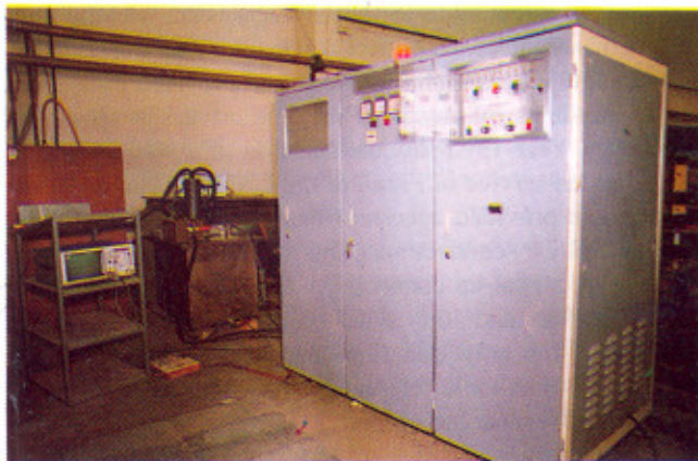
5MW Klystron test station showing the klystron modulator and high voltage tank (visible at back).
