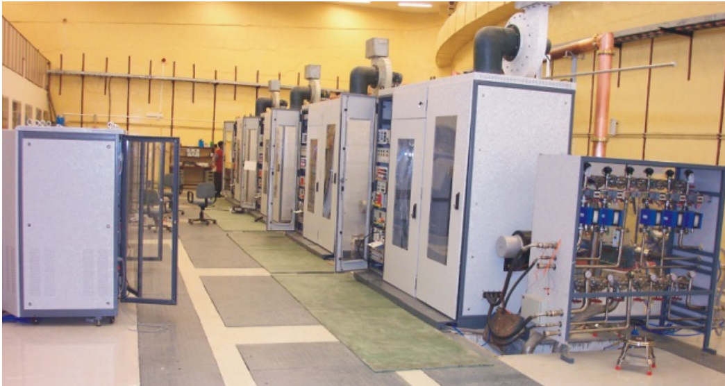
Fig. T.2.2 505.8 MHz RF Transmitters
