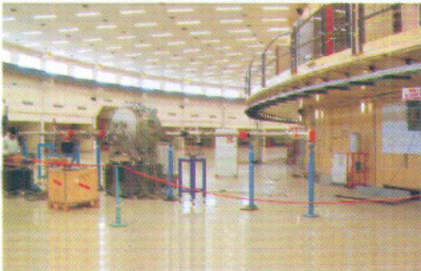
Assembly of High Resolution X-Ray Diffraction Beam Line (BL-12) in Indus-2 Experimental Hall
