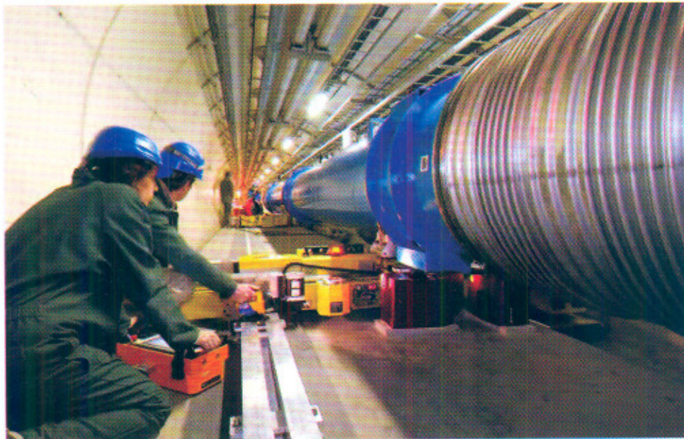
High precision jacks delivered by our Centre to CERN being installed in LHC tunnel
