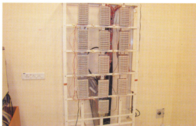
Fig. I.3.15: MDF commissioned at SCRF building
