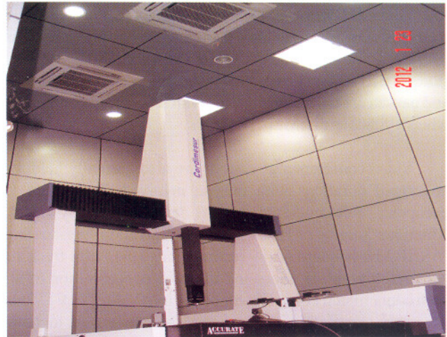
Fig. I.5.5: View of CMM Hall showing cassette air conditioning units and insulated wall cladding
