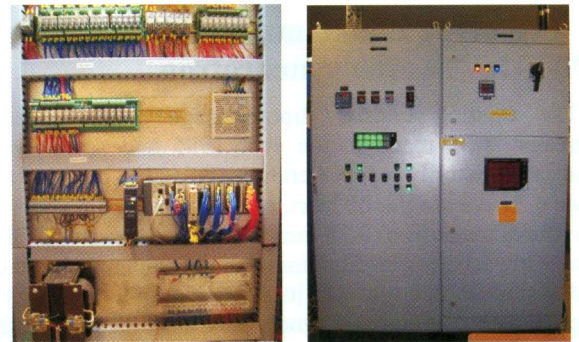
Fig. A.10.2: DAQ system and chiller panel
