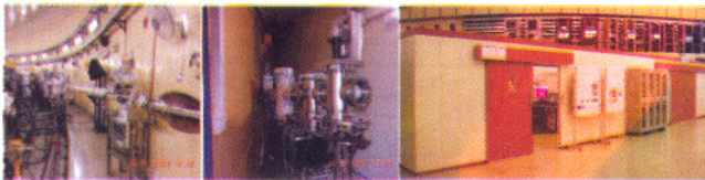
Fig. A.2.2: Some photographs of installed components at X-DBL; beamline portion inside Indus-2 tunnel (left), beamline portion inside radiation shielded hutch (middle) and beamline hutch in the experimental hall (right).
