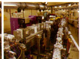
Fig.A.1.3: Undulator U2 installed in LS-3
