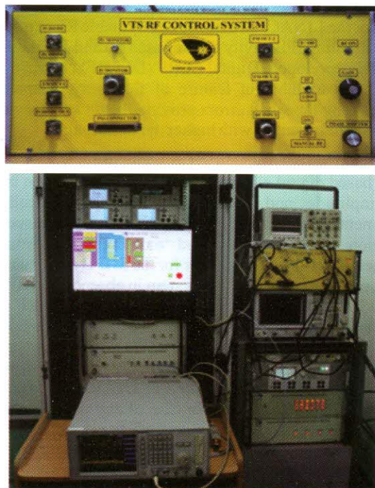
Fig A.18.1: 650 MHz LLRF system installed at the VTS control room.
