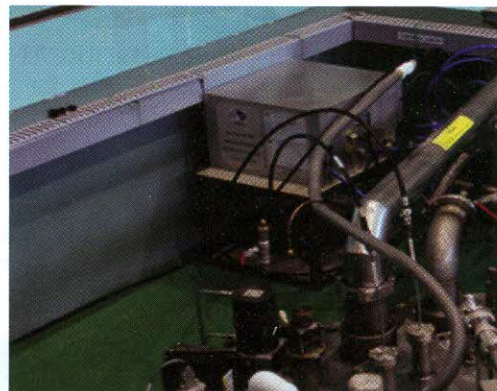
Fig. A.18.2: 650 MHz, 500 W, SSPA installed at the VTS pit
