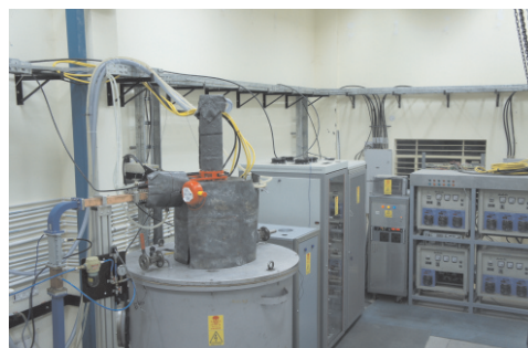
Fig. A.10.3: Microwave system. Klystron, waveguide, tank, PFN cabinet, power supplies
