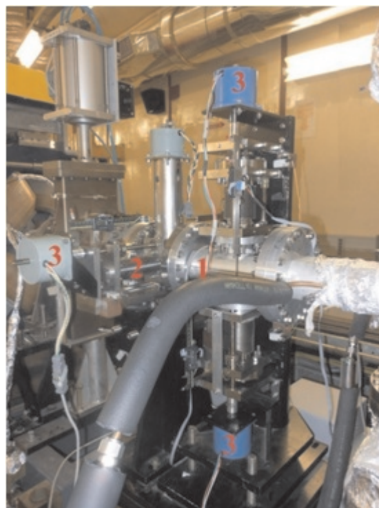
Fig.T.3.7: Vertical and horizontal scrapers in the ring, 1) vertical scraper; 2) horizontal scraper; 3) stepper motors for vertical and horizontal movement of scraper blades
