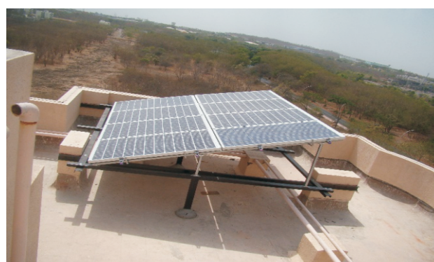
Picture I.2.2: Vindhya Tower Solar PV modules
