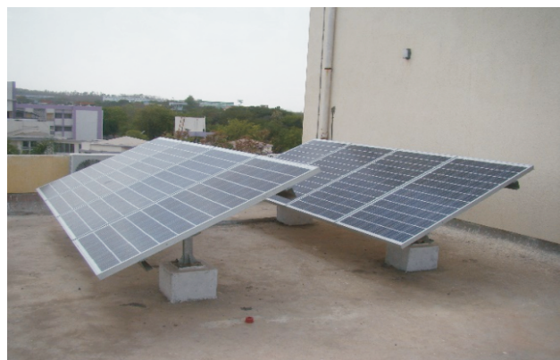
Picture I.2.1: DJ Guest House Solar PV modules
