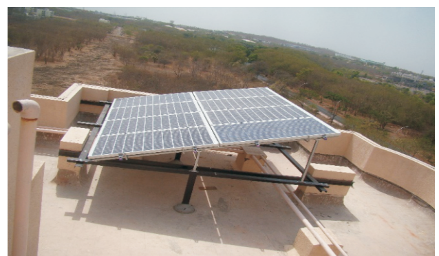
Picture I.2.2: Vindhya Tower Solar PV modules
