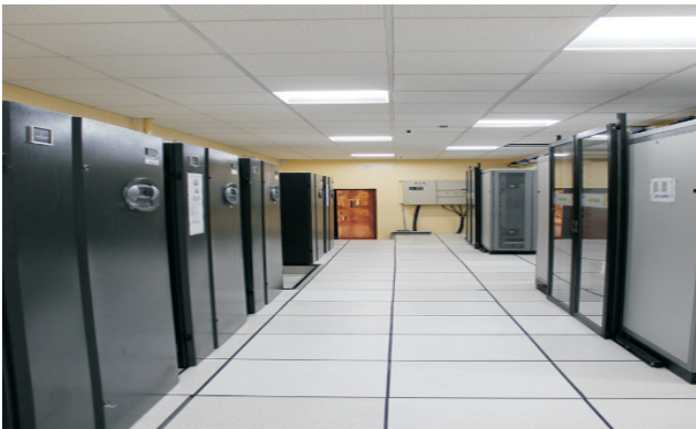
Picture I.1.3: View of Data Centre Hall – A.
