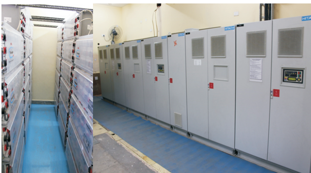
Picture I.1.4: View of UPS and Battery Setup for DCH-A.
