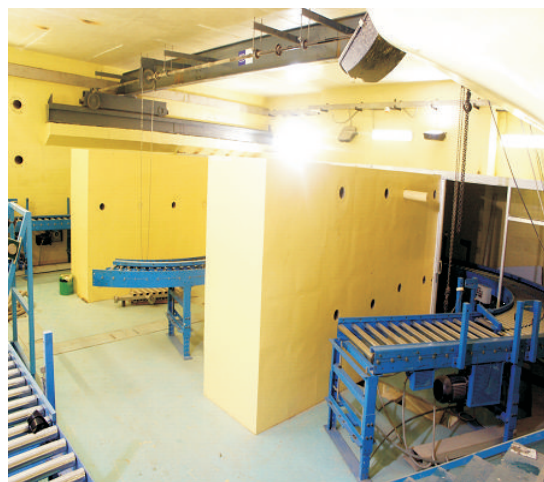
Fig. I.1.4: Localised shielding created for linac in ARPF building
