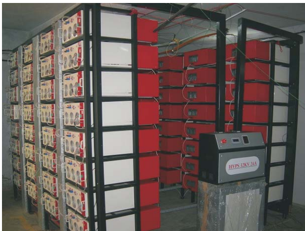
Series connected DC-DC power modules of -36 kV, 24 A DC power supply.
