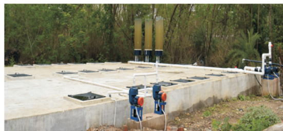
Sewage treatment plant in the technical area.
