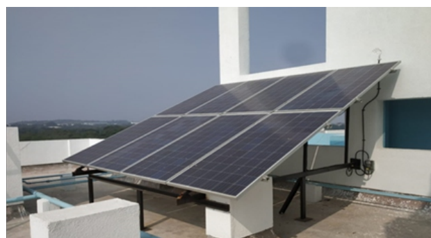
Fig. I.2.3: Solar panels of the commissioned 2 kWp off-grid solar power system.
