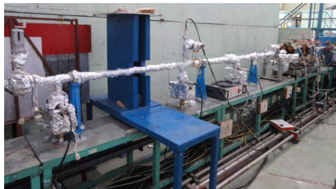
Fig. A.8.1: Photograph of newly installed vacuum system of TL-2 (Indus-1 hall).
