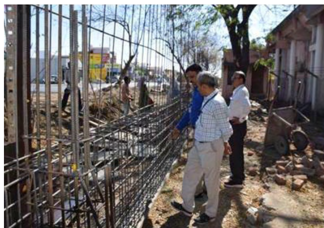
Team of judges inspecting the civil construction site for debris management and general cleanliness.
