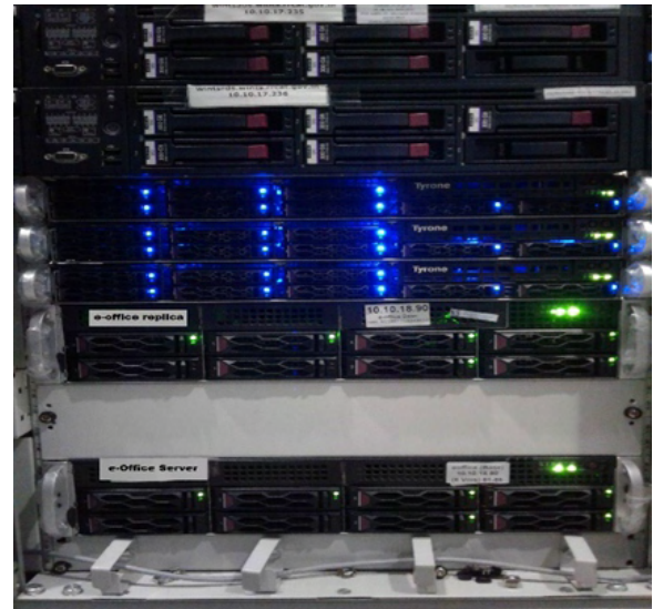
Fig. I.1.2: Photograph of e-Office servers commissioned in DCH-A.
